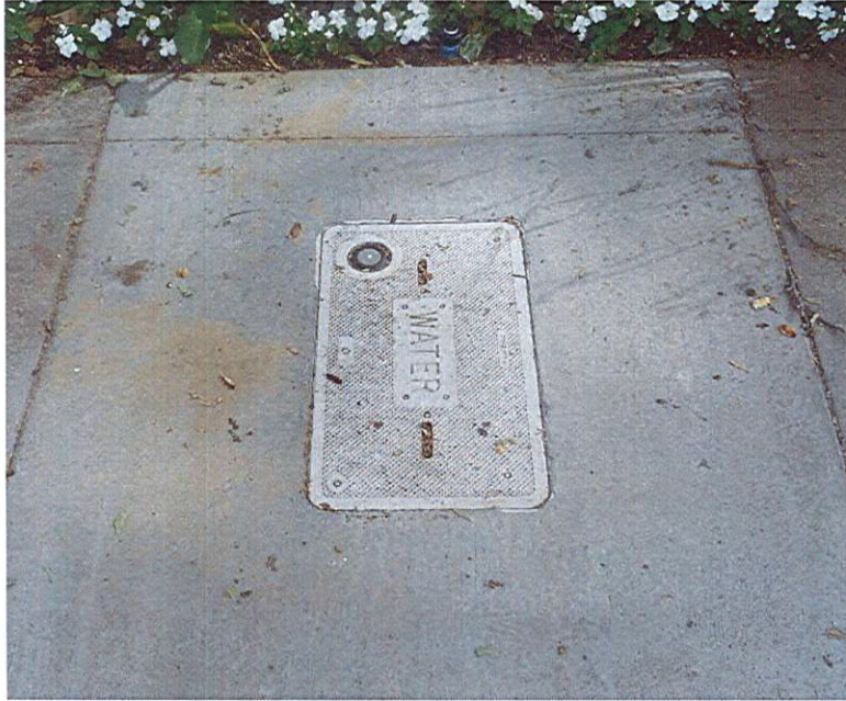
Meter box in the sidewalk
